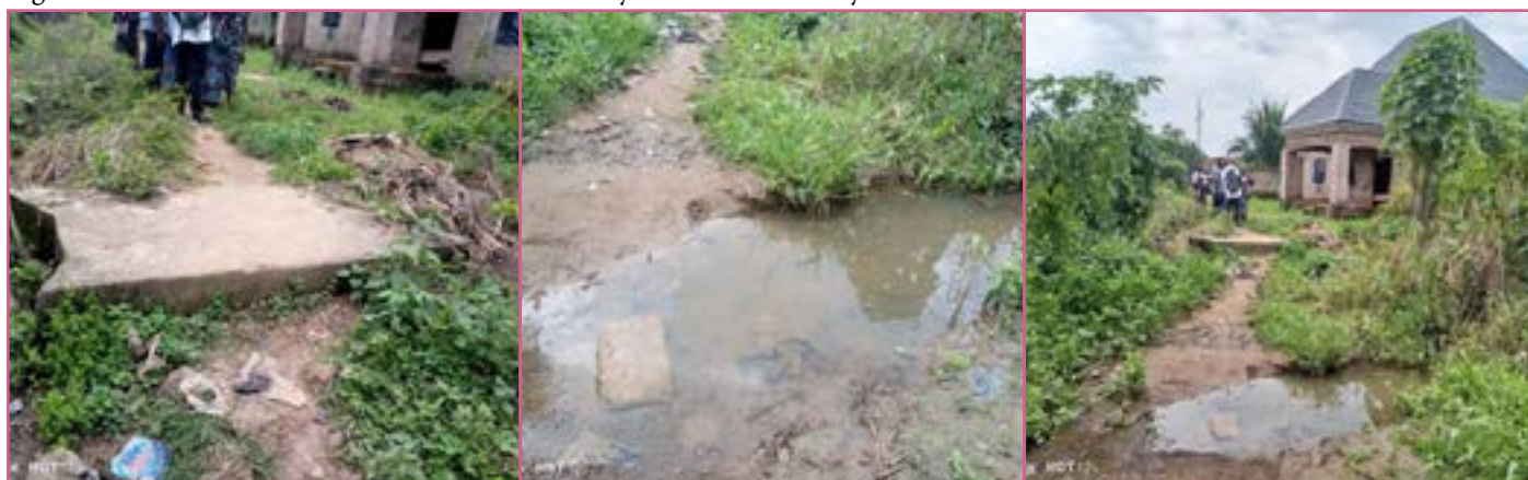
Figure 8 Old Ibe Abbah Culvert constructed far away from the water way and rendered redundant
