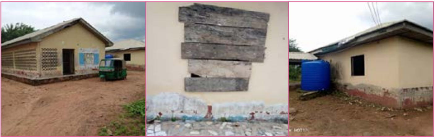
Figure 2 Dilapidated and Poorly Equipped Nochele Health Centre, Ndeaboh.
