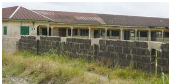
CCSS Biogbolo. No Rehabilitation or Repairs
