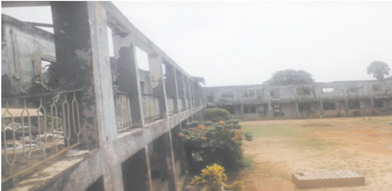
Dilapidated Board Complex at Ministry of Higher Education
