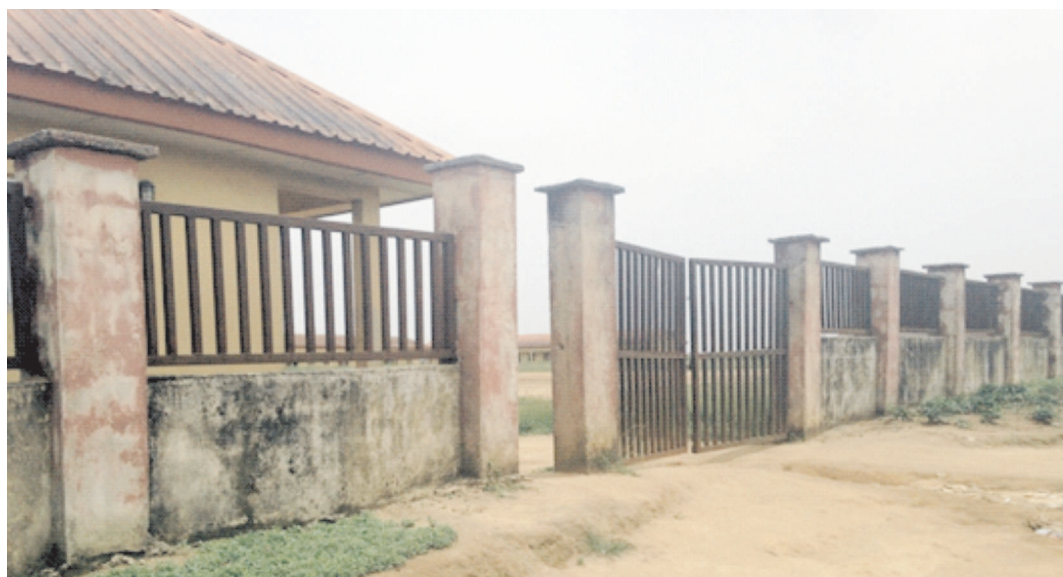
Old perimeter fence at the special education center, Itiam etoi, uyo
