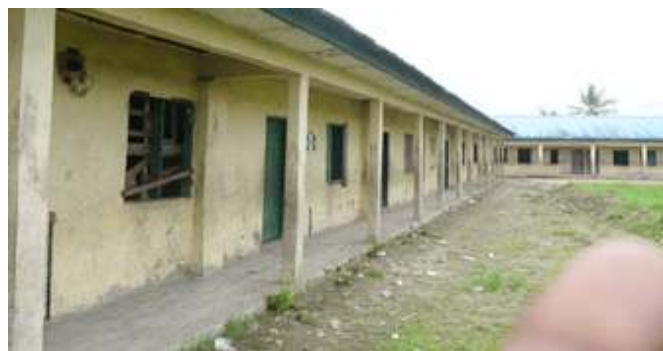
CSS Okaka. No Rehabilitation or Repairs
