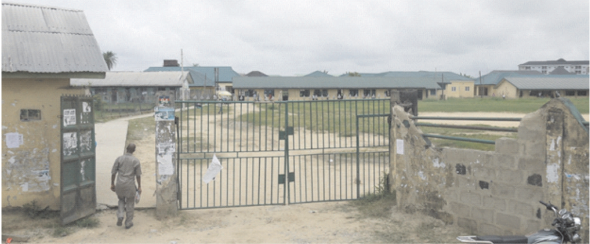
Premises of St. Jude's Girls' Secondary School Amarata. Available space is large enough to contain sports facilities but none was seen at the time of visit.
