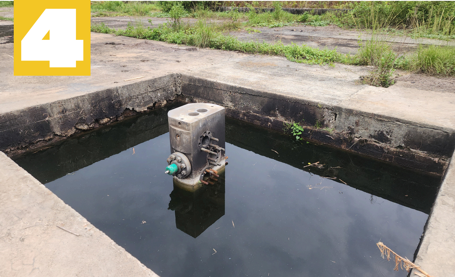
Non-decommissioned well head. A common sight in many oil bearing communities in the Niger Delta
