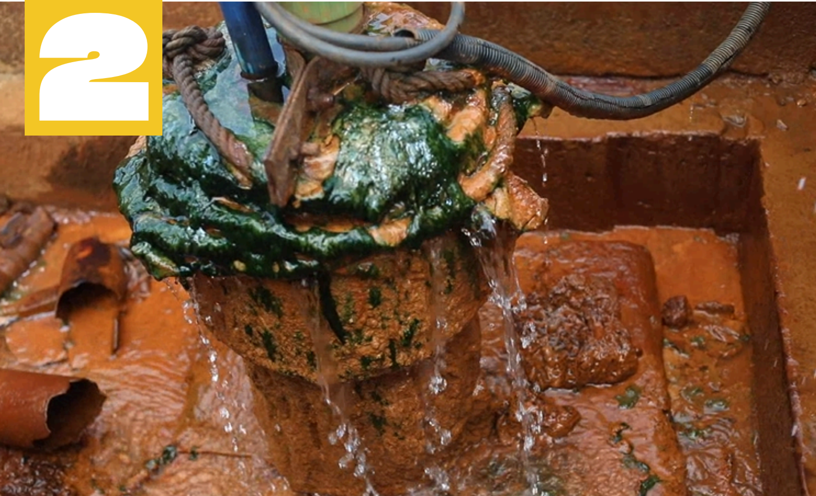
Water boreholes in Bille are leaking under intense underground gas pressure
