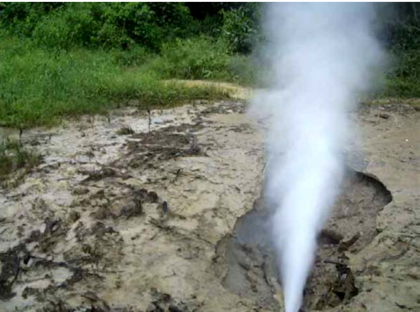
Oil & gas leakage from Agip pipeline in Ikarama July, 2010
