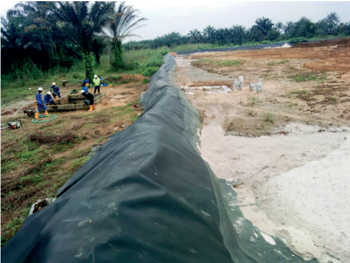
Workers on a remediation site without any warning sign or indication of what is going on there
