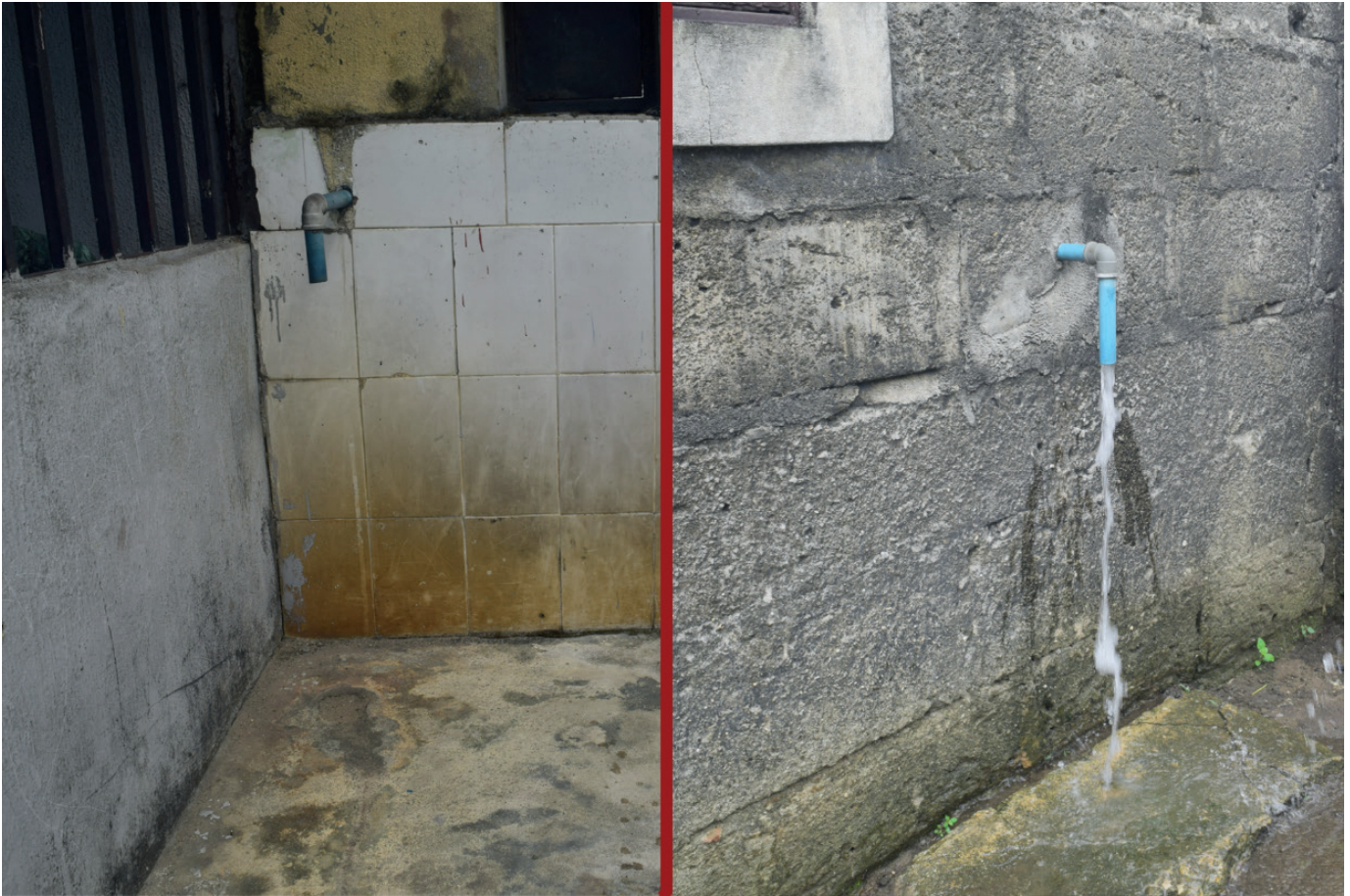
Some boreholes with evidence of hydrocarbon in the water without any warning signs
