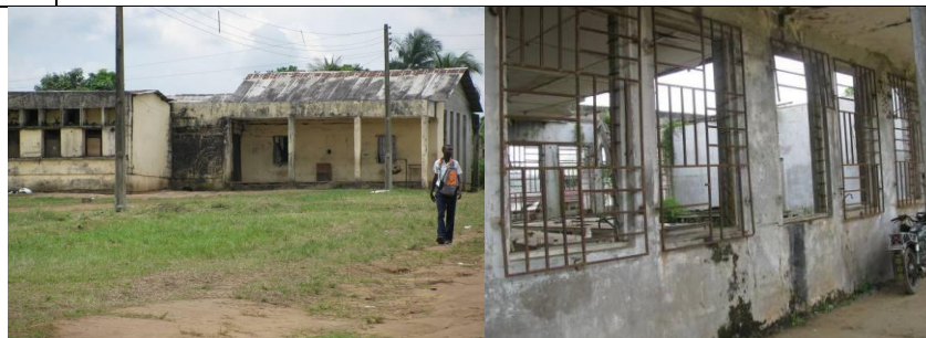
Hostel Building and Physics Lab. At Technical College Abak as at October 2010.
