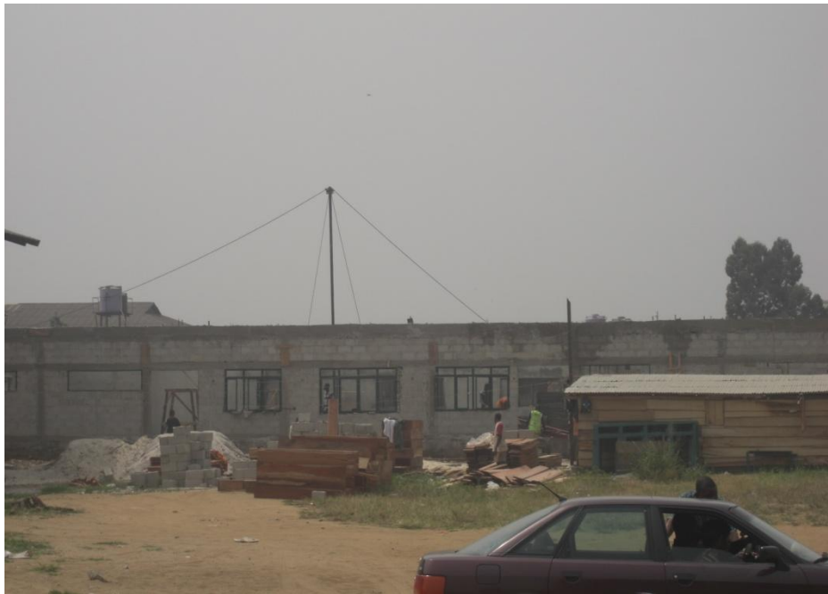
St. Andrews Model Primary School, Port Harcourt, under construction as at January 2011
