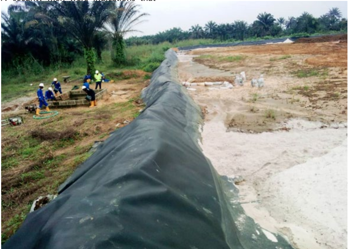
Workers on a remediation site without any warning sign or indication of what is going on there
