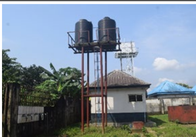
Non-functional water project in Ogale
