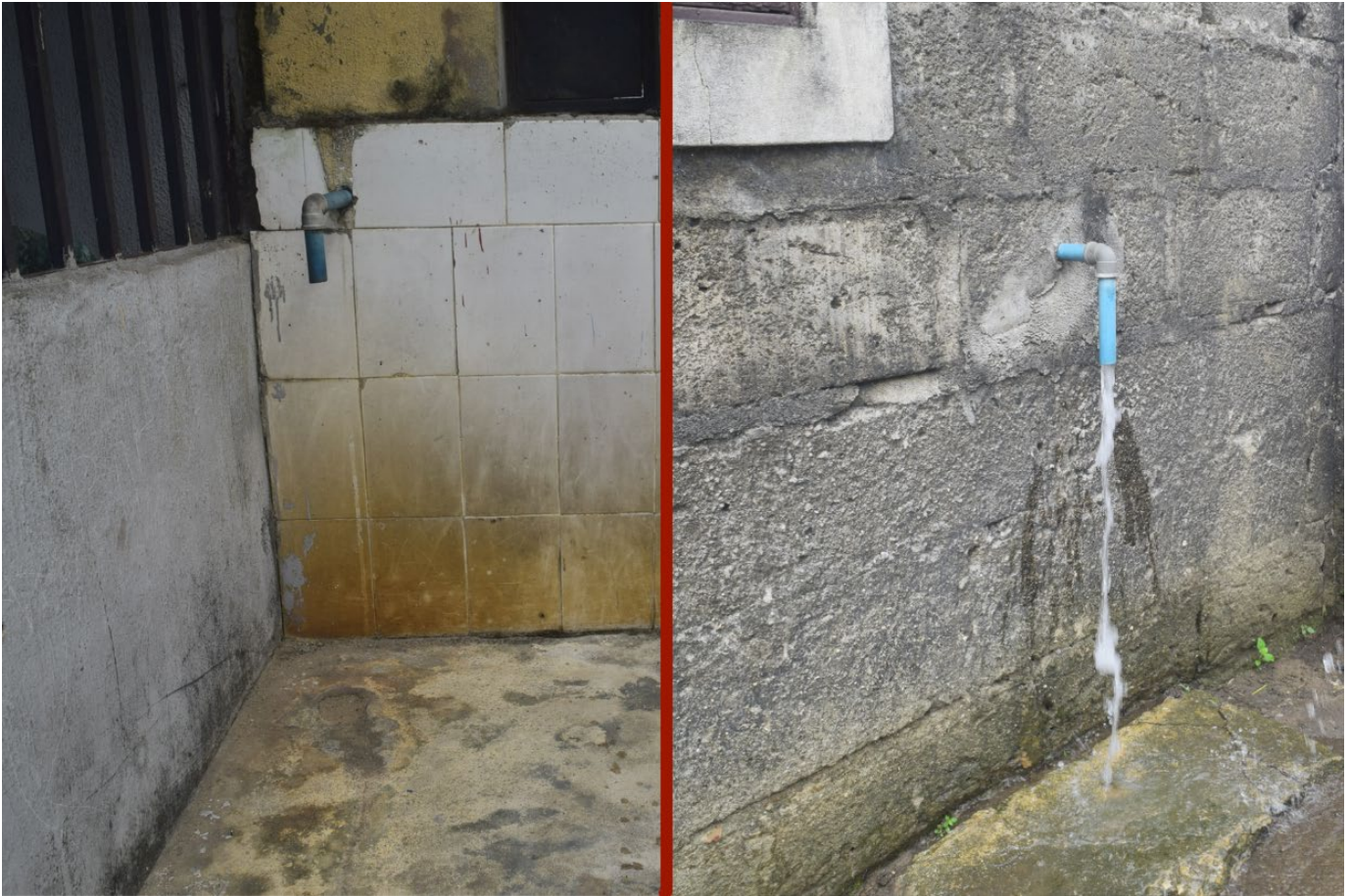
Some boreholes with evidence of hydrocarbon in the water without any warning signs
